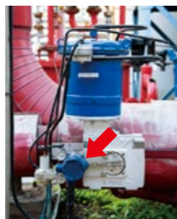
A smart valve positioner attached to an Azbil valve used to regulate hydrogen pressure in soda electrolysis equipment.
